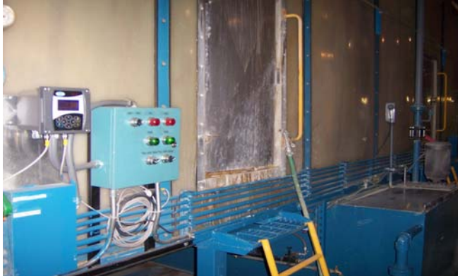
Photo of Analyzer on left, electrical panel in middle and sensor on far right in tank 4, solenoid not shown.
